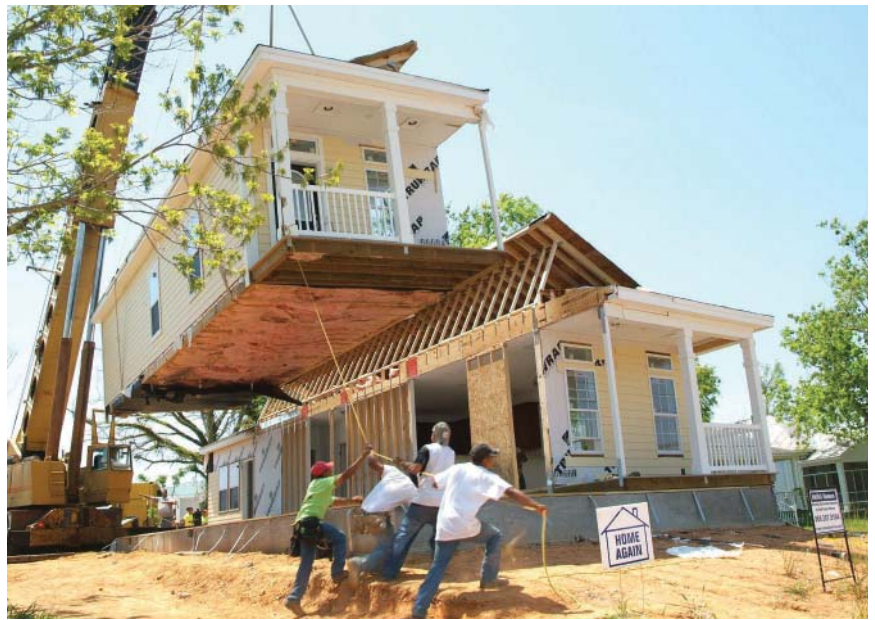
Local residents participate in a houseraising financed by ECDI/Hope Community Credit Union in Mississippi after Hurricane Katrina. The local credit union was instrumental in helping storm victims recover from the disaster.
